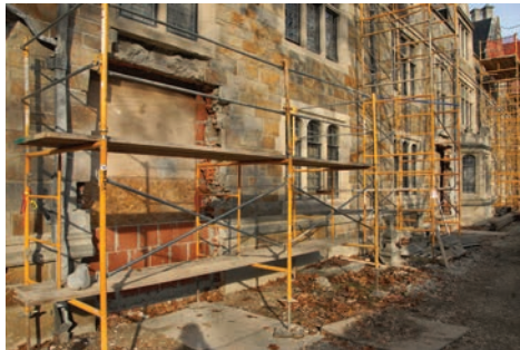
The Law School community celebrated the reopening of the Lawyers Club on August 19, 2013, following a $39 million renovation that transformed the interior while keeping the iconic exterior largely unchanged.
